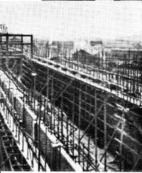
Construction of China's first automobile plant is now in full swing in the Northeast
