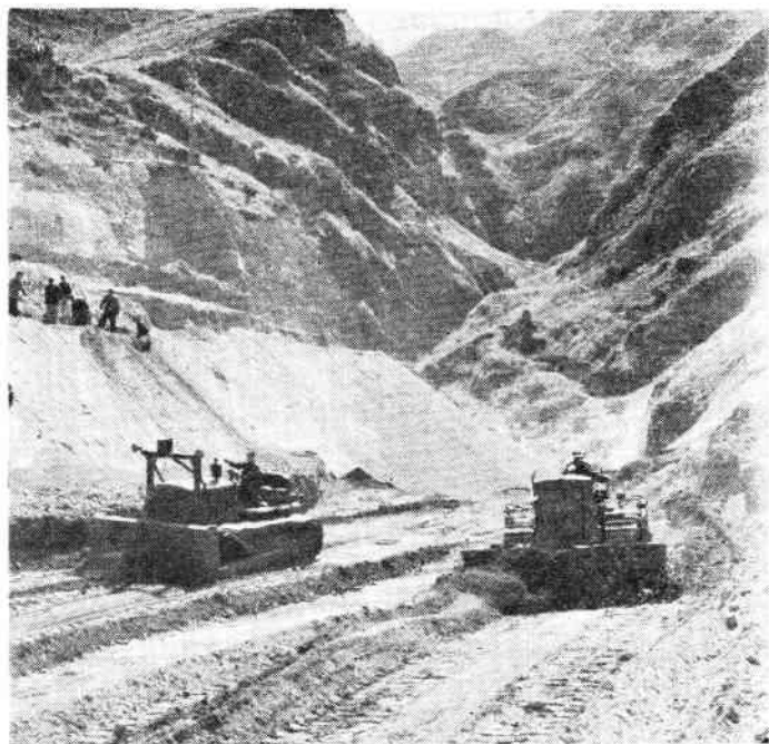
Work on another stage of the Kuanting project has commenced. Bulldozing the site of the power station which will tap the waters of the reservoir
